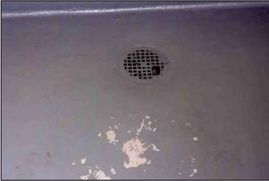
Figure 5 Shower Stall Drain and Floor
