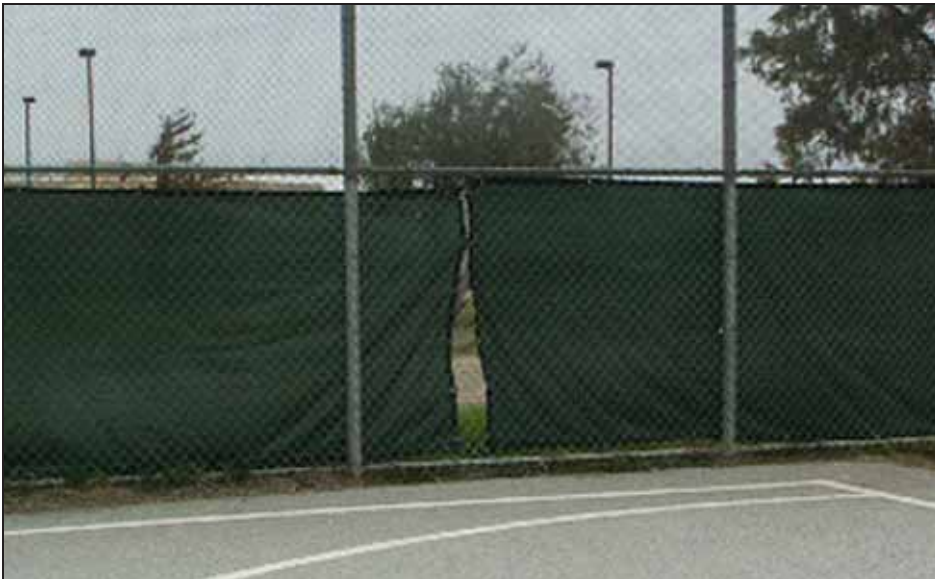
Figure 19 Close-up of Gap in Security Fence
