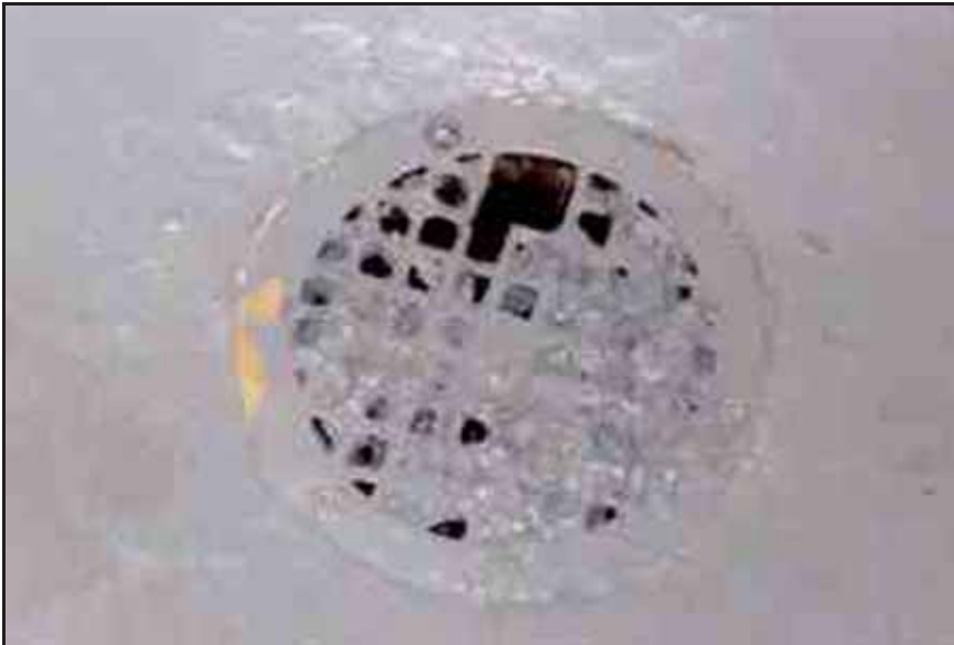
Figure 6 Close-up of a Shower Drain
