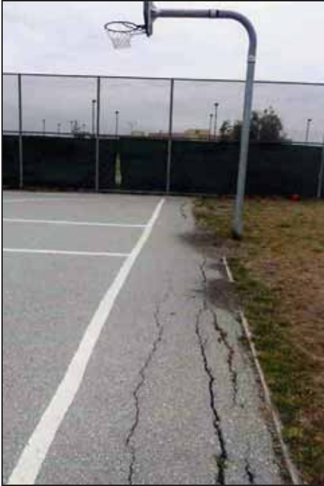
Figure 11 Typical Asphalt Condition in Courtyard
