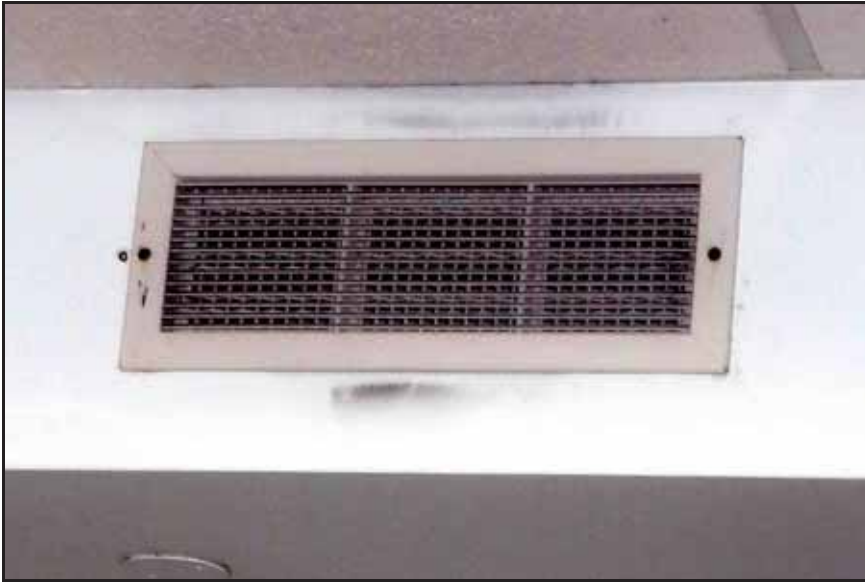
Figure 9 Typical Air Vent (from Courtroom)
