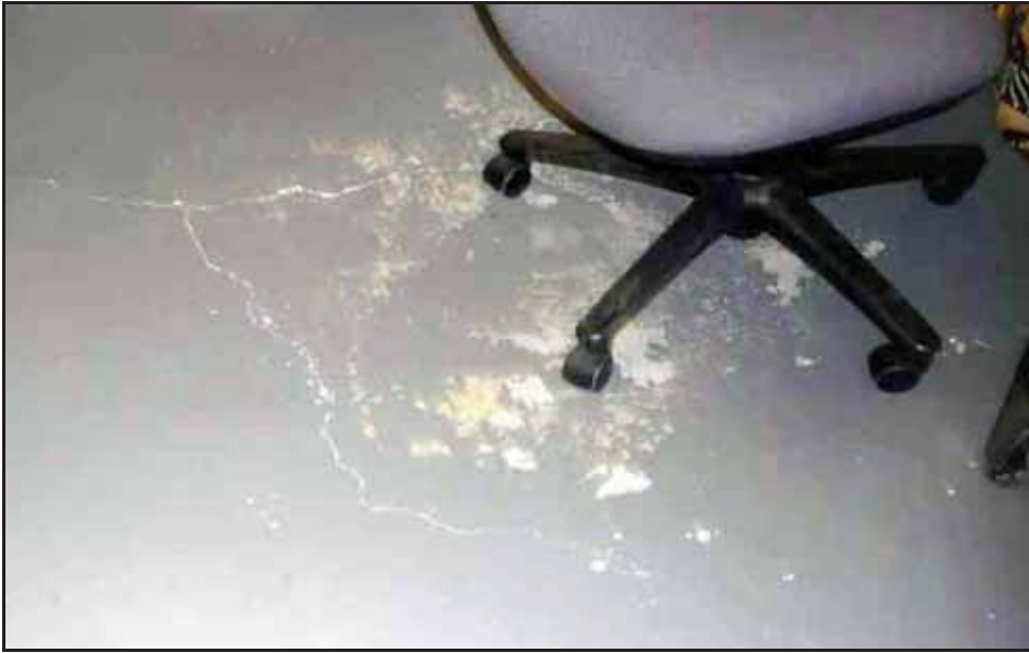
Figure 1 Example of Poorly Maintained Concrete Flooring
