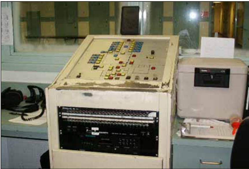
Figure 10 Security Control Panel
